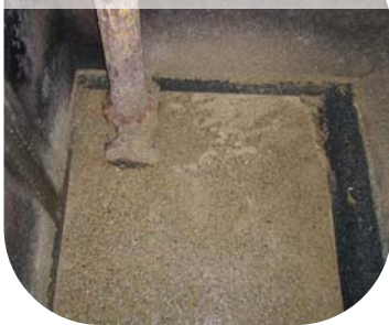
Ft. Collins, Colorado Before: 4" grease
