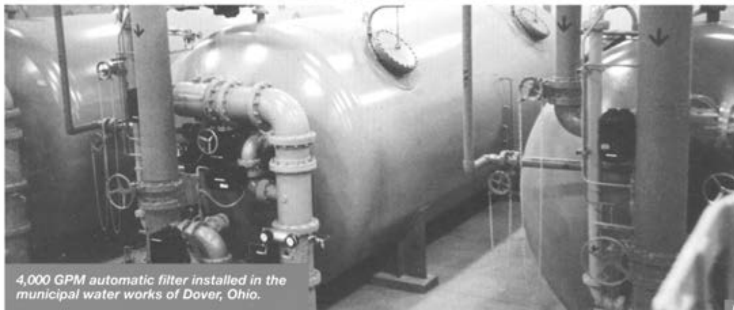
This is an example of the 1.5 MGD municipal filter installation with air/water wash, by Hungerford & Terry.
