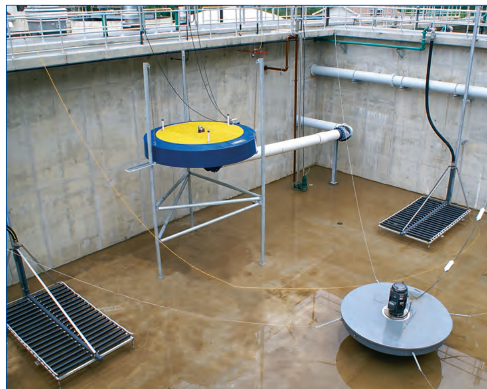
Full floor coverage diffused aeration is standard, optional retrievable diffusers are shown.
