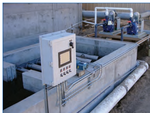
The rotating backwash system is PLC controlled.
